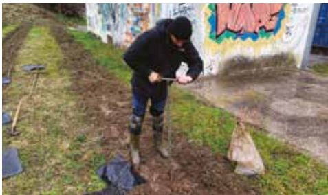
2. Excavation of the hole using manual mechanical equipment or a motorised auger
